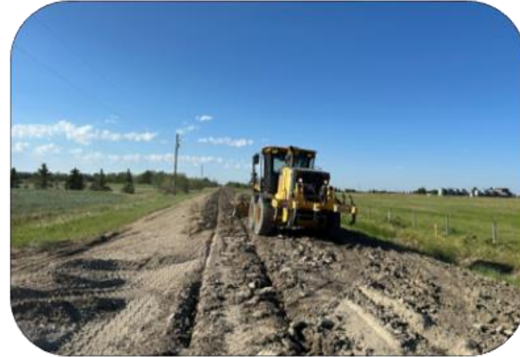
Rge Rd 261 – Twp Rd 554 to Hwy 642
